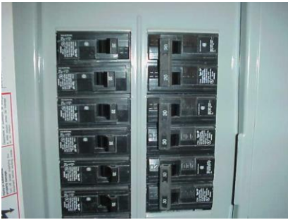
Circuit Breaker Box
